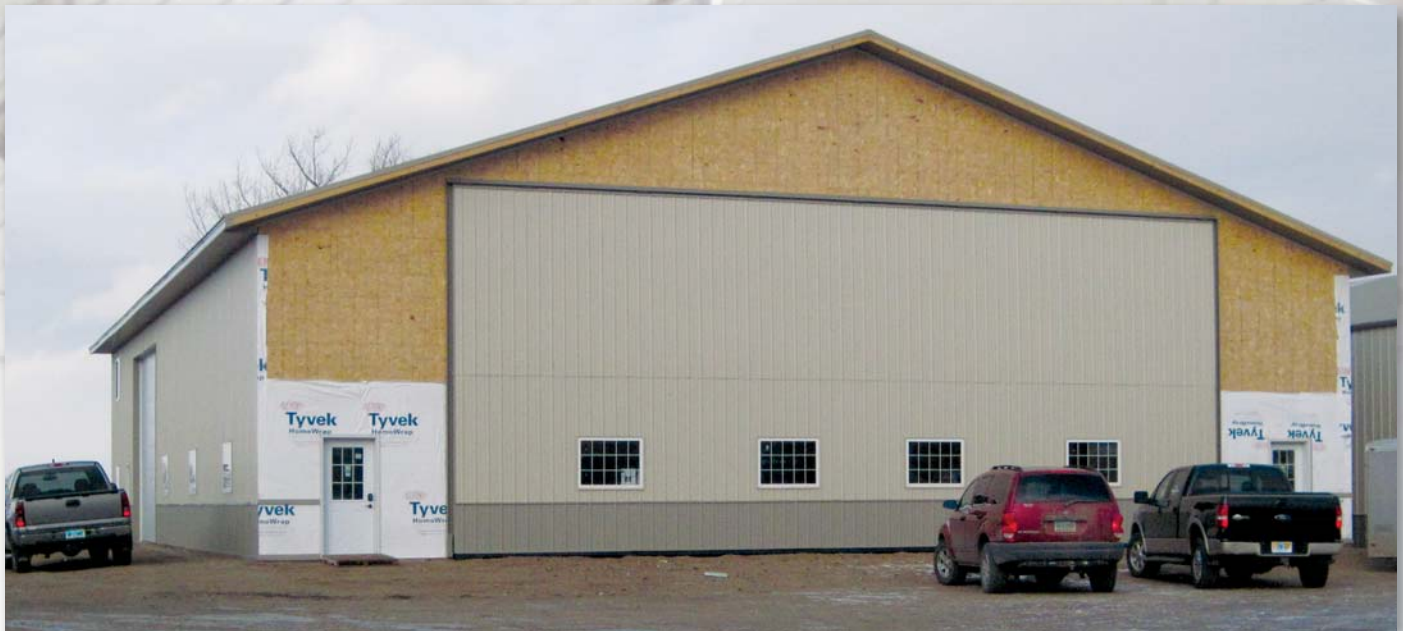
A new farm shop is under construction at LeClerc Farms near Oakwood, N.D.
