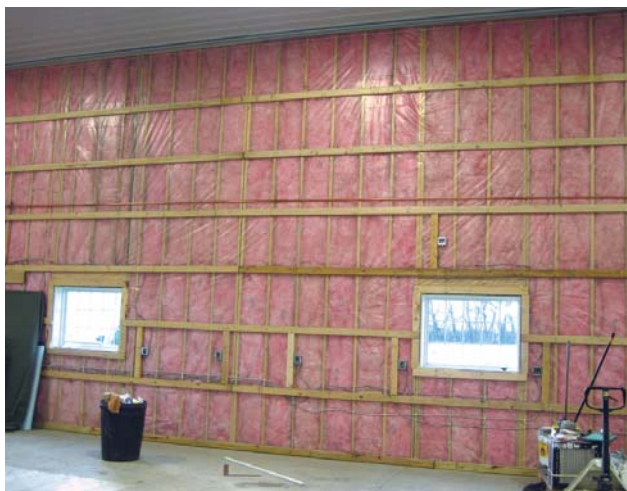
A well-insulated shop is one of the most cost-effective ways to cut energy costs and help heating systems operate more efficiently, as shown in the LeClerc shop.
