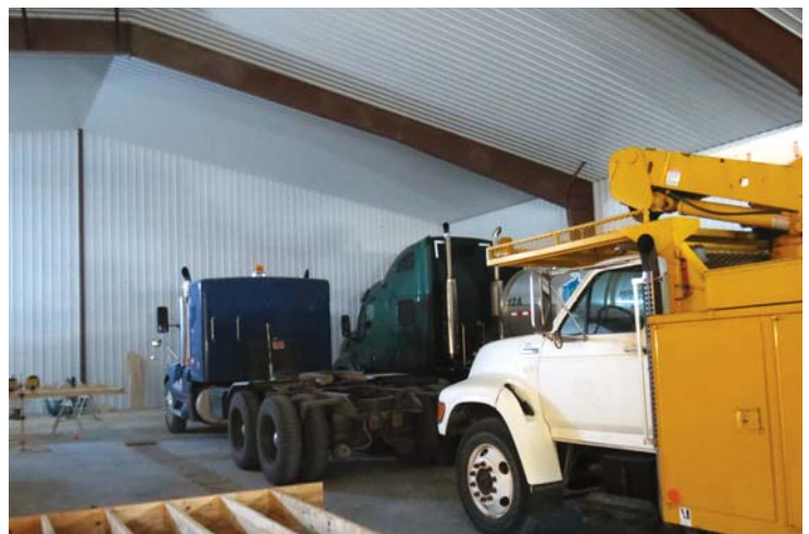
The Vettel shop uses spray foam ceiling insulation to reduce heat loss and keep work areas at a comfortable temperature.
