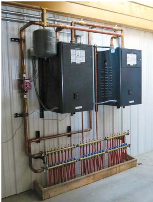
By installing a 62-kW electric boiler in his new shop, Ernie Vettel of Caledonia, N.D., is set to enjoy a warm workspace and Nodak's low off-peak electric heating rate.
