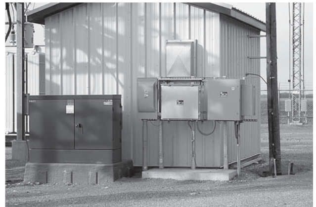
Substation control equipment located at the Coleman substation south of Grand Forks.
