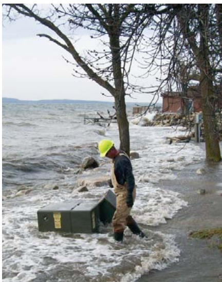
Lead line worker Cory McKelvey prepares to remove a transformer in the Devils Lake area.
