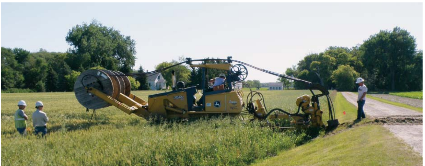
North Plains Utility Contracting works on installs underground lines near a farm south of Grand Forks.
